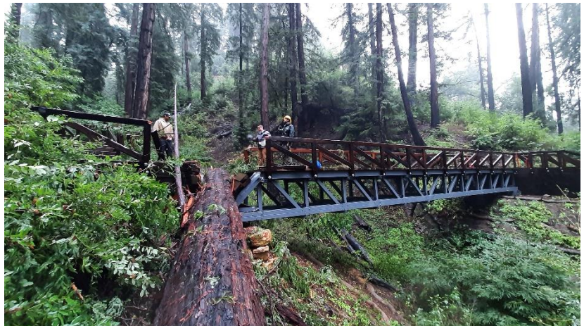
Recent severe storms caused significant damage to throughout the park system, including to this bridge in Pfeiffer Big Sur State Park. Photo by California State Parks.
