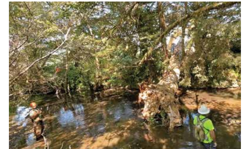
The Yurok Tribe Construction Corporation and Fisheries Department installed large pieces of wood in stream channels to improve habitat for salmon and other aquatic species.
